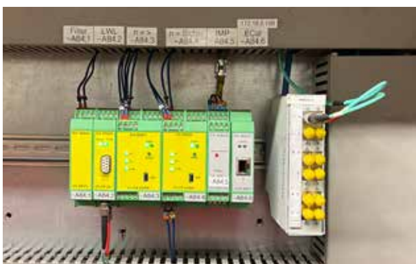
Function modules of the U-ONE universal encoder system in the switchboard.
