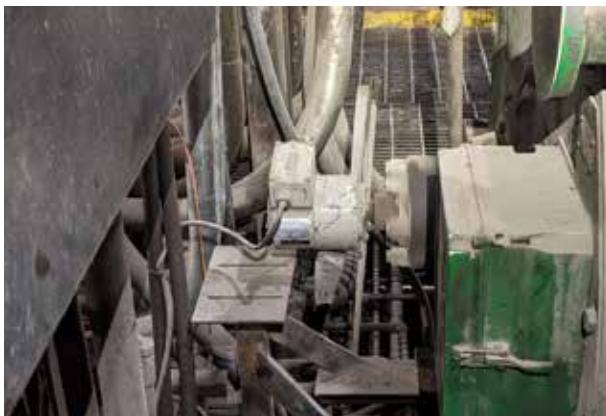
The basic unit of the U-ONE universal encoder system at the installation site.
