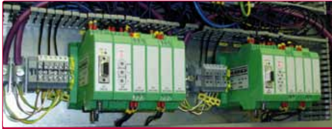
U-ONE® up close: electronic function modules mounted in switch board.
